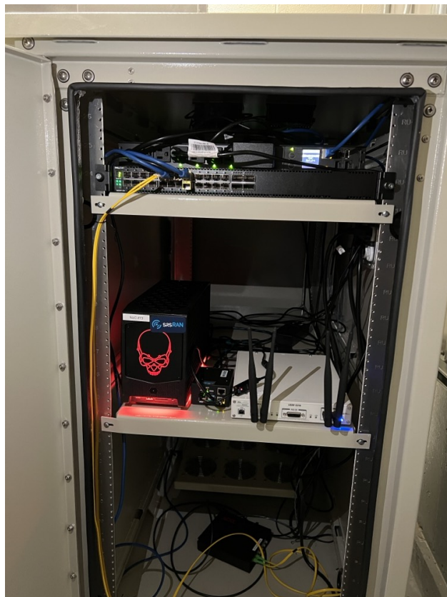
Figure 1.8: The cabinet installed for the outdoor CBRS-based xG testbed.
