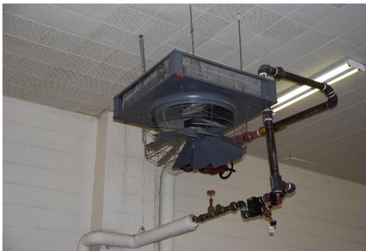
Image #9: Air Circulation System in Old Powhatan Housing Buildings
