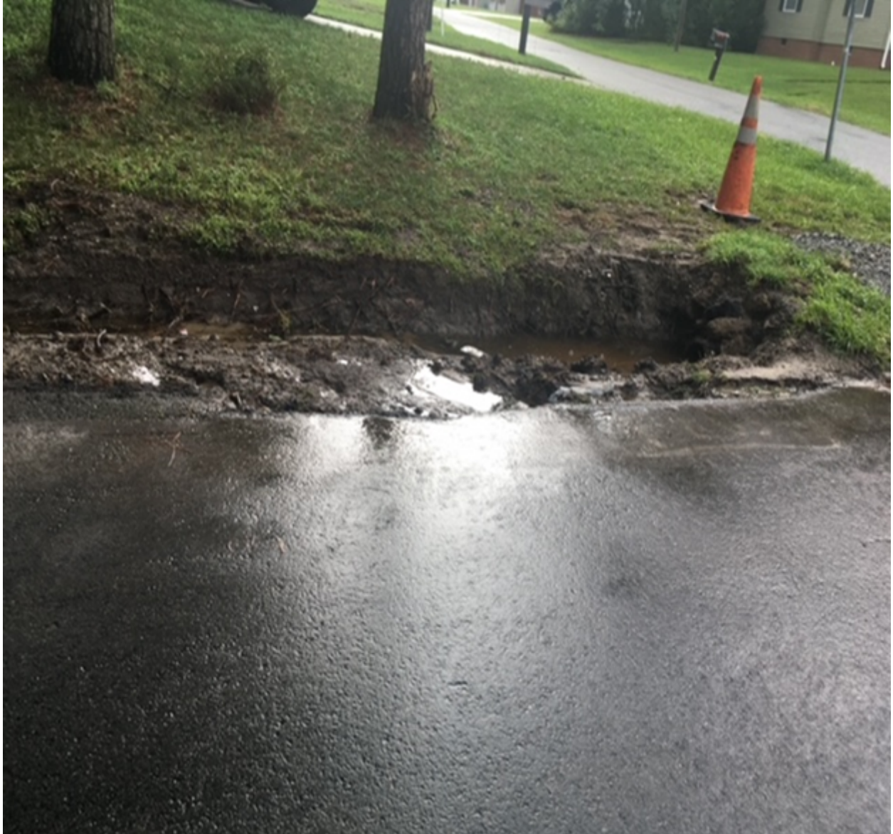
Caption: Soil Erosion near the John Street outfall in Pughsville. (Photograph provided by Carolyn White).
