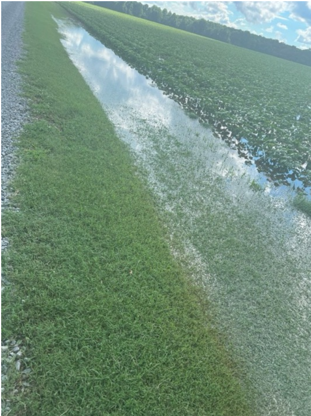
Caption: Poorly maintained drainage ditches in Oakland-Chuckatuck. (Photograph provided by Leslie King)
