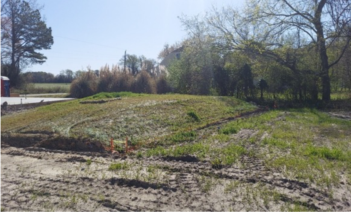
Alternative sewer systems which have been approved for newer construction contribute to flooding because of the elevated mounds which cover these above ground installations. Water channels off these mounds and can flood out lower lying adjacent properties. (Photograph provided by Mary Hill).
