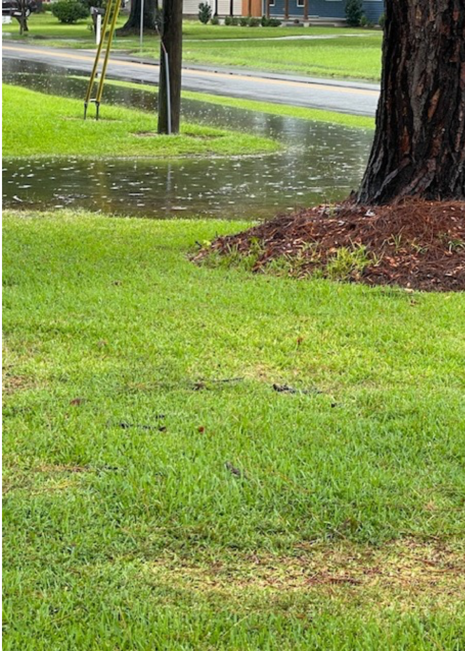
Caption: Storm sewer overflowing during moderate rain events. (Photograph provided by Carolyn White)
