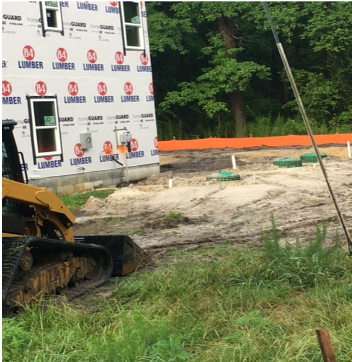
Caption: Above ground sewers permitted for newer construction in historic African American community of Pughsville. (Photograph provided by Carolyn White).
